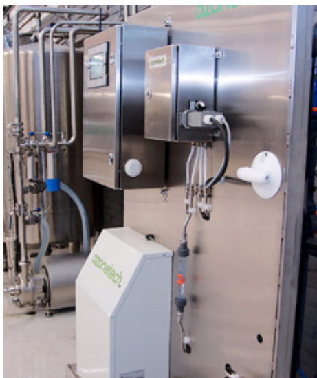
The RENA Vivo A-series is integrated into the existing CIP system.
